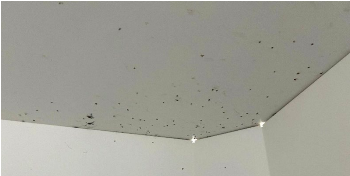
Figure 22. Insect Infestation in Shower Facilities; Observed January 21, 2026
